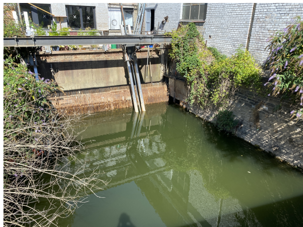
Figure C.4: Mery Site - Kaplan turbines & Bypass
