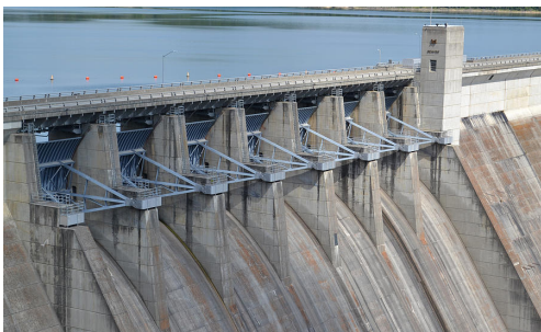
FIGURE 1.2: Beaver dam (US) – gated spillway (finartamerica, accessed in June 2023).
