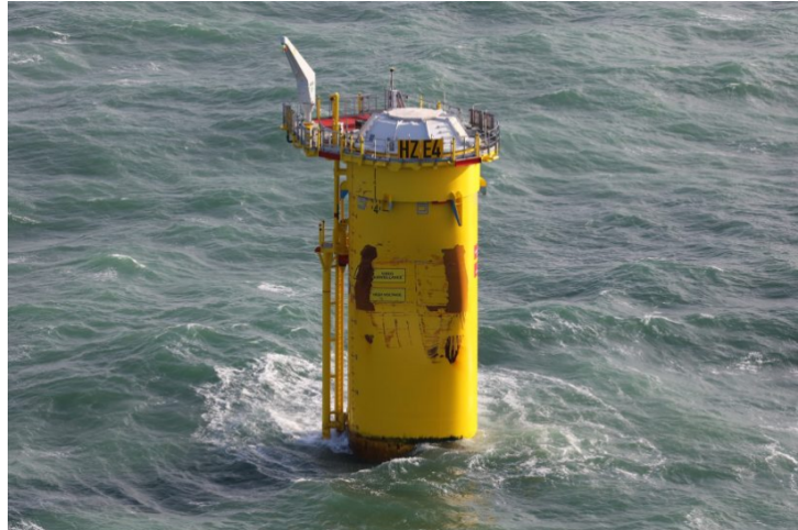
Figure 1.2.: Damaged monopile foundation from an impact of a drifting cargo vessel (Dutch North Sea). From ( Margientimmer, 2022 )
