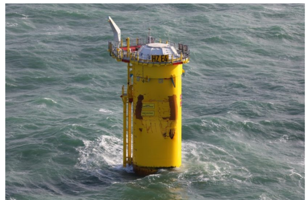
Figure 1. Damaged monopile foundation from the impact of a drifting cargo vessel (Dutch North Sea) - From (Hollandse Kust, 2023)
